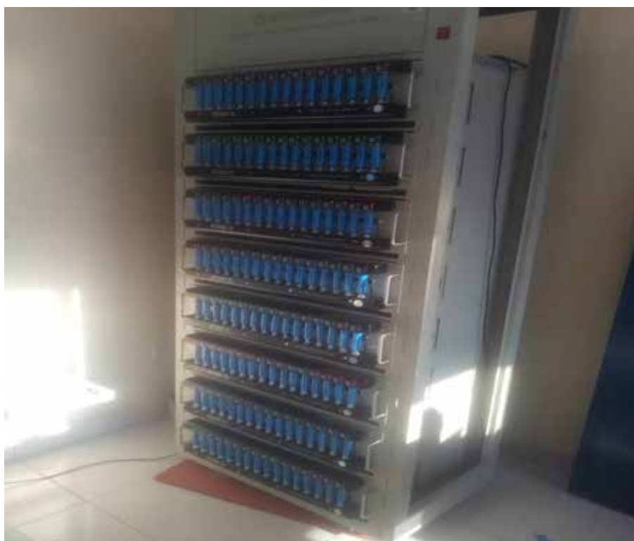
Figure 3: Lithium-ion batteries and charging and discharging cabinet at the Enviroserve facility
